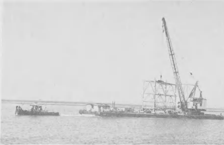
ONE OF two structures that support No. 3 Finger Pier's free-standing loading arms is transported by a Raymond barge from the assembly area near the Gasoline Docks to the pier's breasting island.
